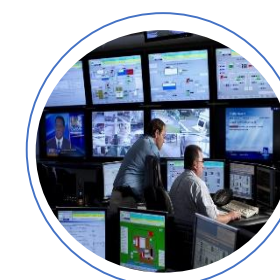
CONTROL ROOM & UPKEEP MANAGEMENT
